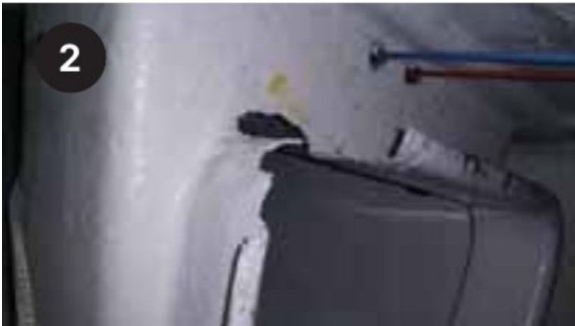
Picture 2: check the GRP part of the spinnaker chute for damage
