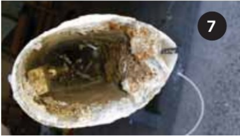
Picture 7: debris and corrosion inside the mast foot
