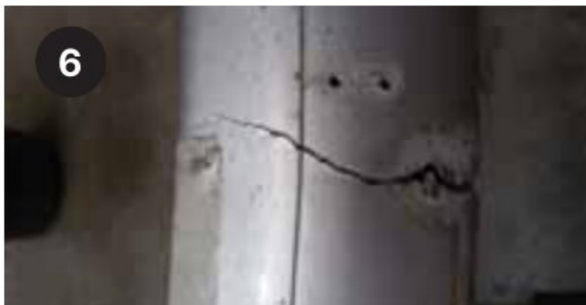
Picture 6: cracking around the mast ram fitting
